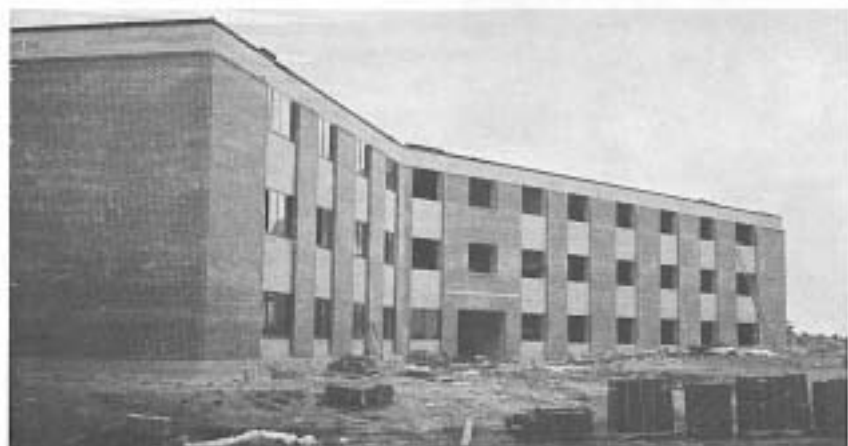
A close-up view of the Bible School building which will be dedicated at next year's annual conference. The ground floor will provide two classrooms for the present and house boys in the left wing. The building is being furnished by individuals and by Ladies Aid groups in the Association.
