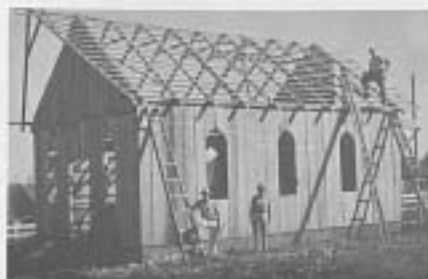
One of our new churches under construction. It is located in Lar Parana, a suburb of Campo Mourao, Parana. Missionary Alvin Grothe is standing on the roof.
