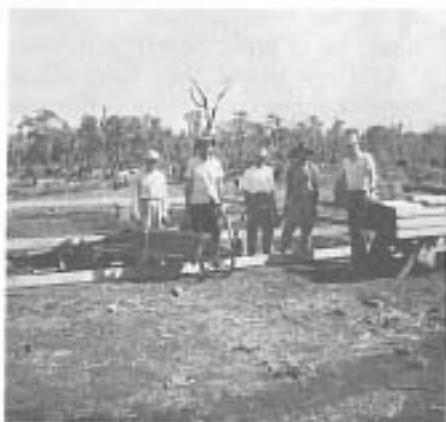
A church with cement pillars and brick foundation is being built in Santo Rei. Here are four Brazilian men of the congregation with Pastor John Abel as construction is beginning. Pastor Abel held several evangelistic meetings in a warehouse and then in a grade school in this new town. Ours is the first church in Santo Rei.
