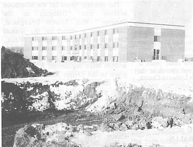
During the excavation of the basement for the new dorm. The present dorm is shown in the background.
