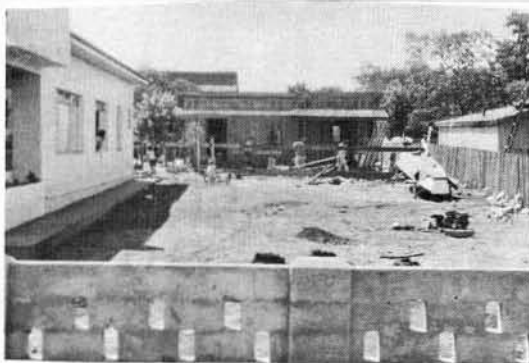
5. Arriving at our new little brick home, we work on wooden rooms out back in order to have room for our family and belongings.
