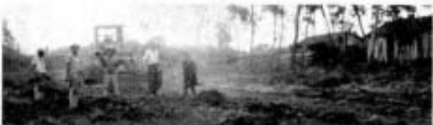
Clearing stumps, bushes and rocks from the front of the lot, Mr. Grothe can be seen to the left of center.
