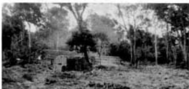
The beginning! Here the trees are being cut down and clearing has begun as the first bricks and lumber arrive. (The smoke is from the burning trees.)
