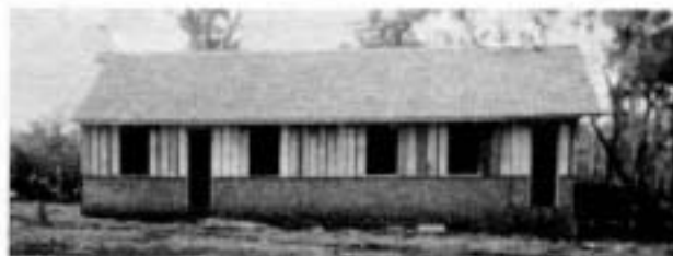
The roof is on. The four thousand tile needed for the roof had to be washed by hand first.
