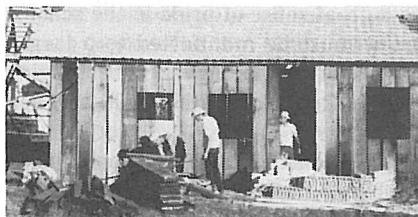
Building the parsonage at Umuarama. The church is to the right of the picture. Calvin Knapp is shown on the roof, and on the ground, left to right, Pastor Vitor, Halvor Knapp and Pastor George Knapp.
